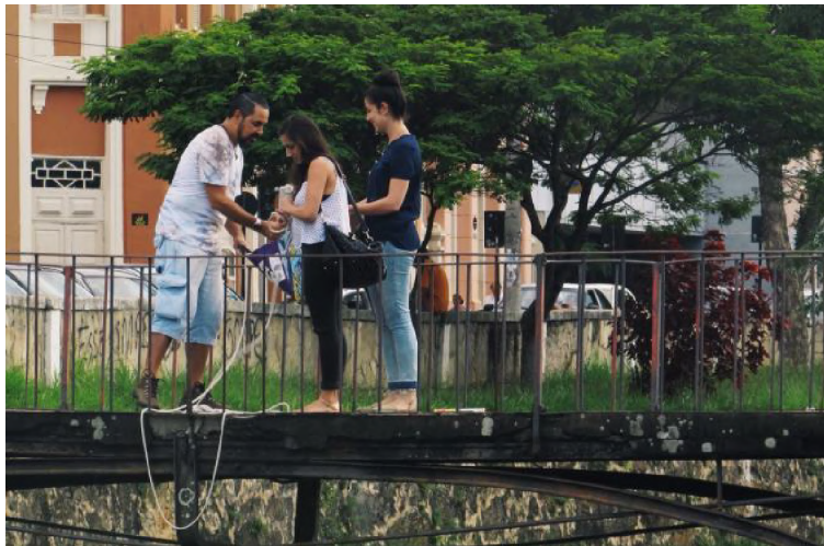
Fig. 12: Team members preparing to install the swing on the Coreto Bridge. Source: Authors.
