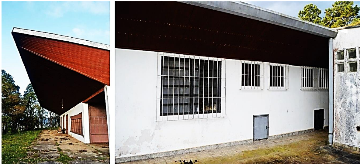
Fig. 7: Inclination of the holes in the north and south elevations.
