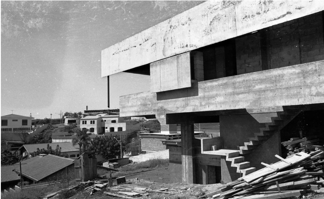
Photo 8. Construction works at Janne Ottoni residence. Northwest façade. Photography by David Ottoni, c.1973.
