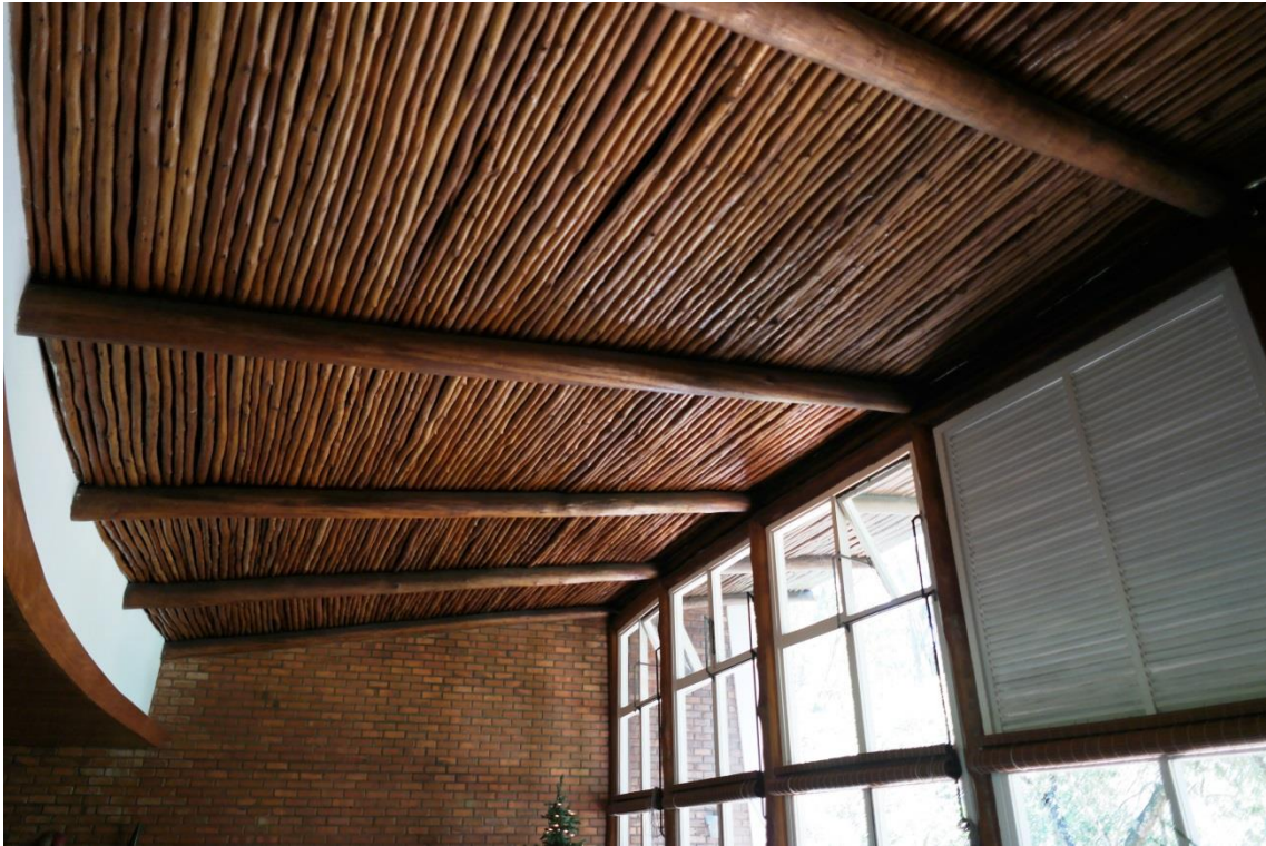
Fig. 6: Roof detail of Lauro de Souza Carvalho House, from Henrique Mindlin. Samambaia, Petrópolis. Source: Silva, 2014.
