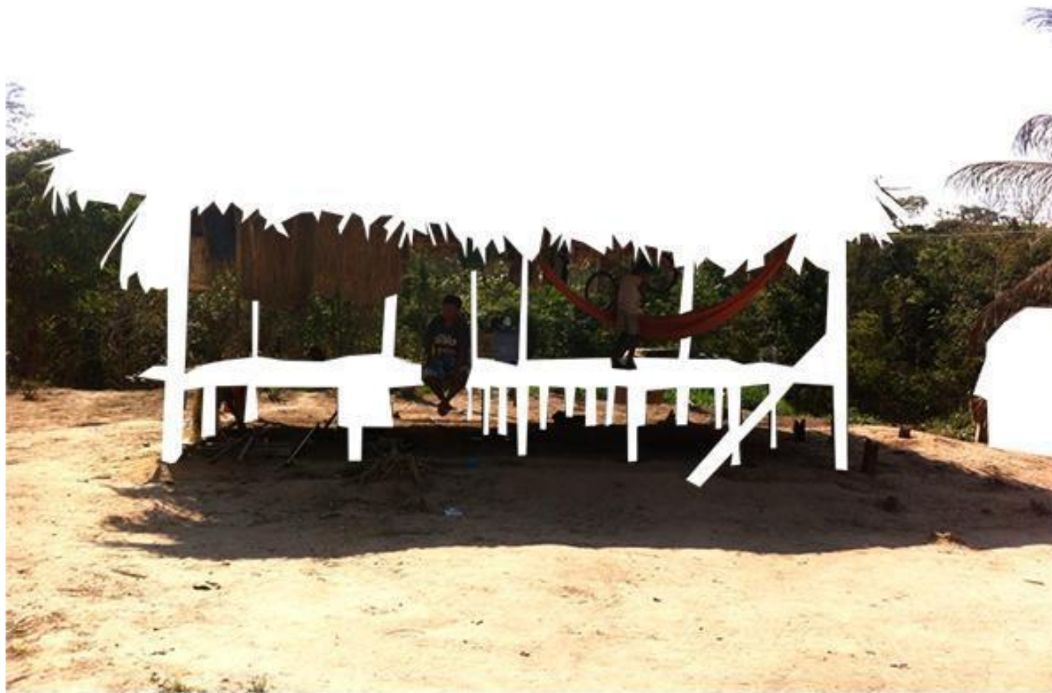
Fig. 6: Photographic record of a house under construction in Mutum village. Source: Mendo, 2022 [photograph, 2016].
