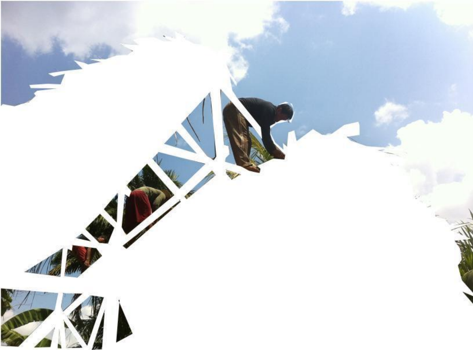
Fig. 7: Photographic record of a house under construction in Mutum village. Source: Mendo, 2022 [photograph, 2016].
