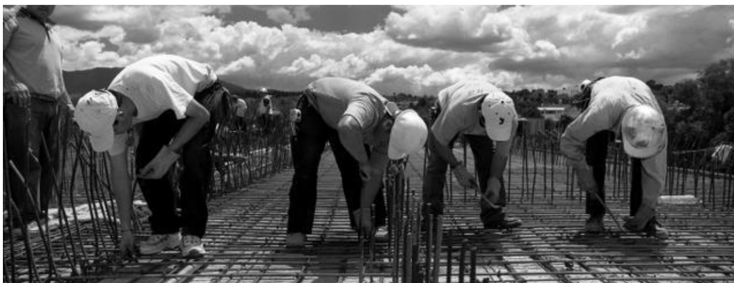
Fig. 2: Construction workers building the elevated highway. Photograph by Ana Lorena Ochoa, courtesy of La Media Luna Productions, 2006. Available at https://lamedialuna.mx/producciones/en_el_hoyo . Accessed on November 9, 2022
