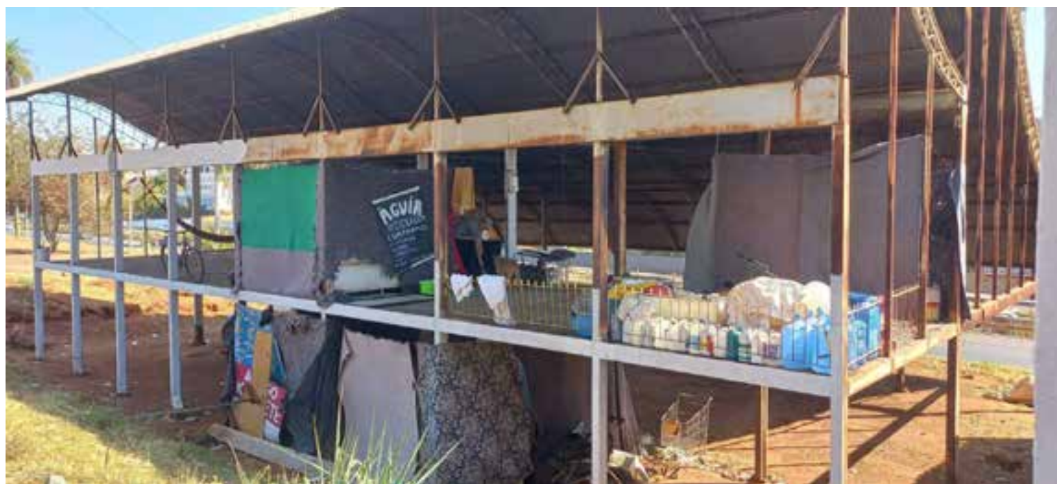
Fig. 2: Ruins of Brazil’s Institute of Architects headquarters – Goiás State. Source: The authors, 2022.
