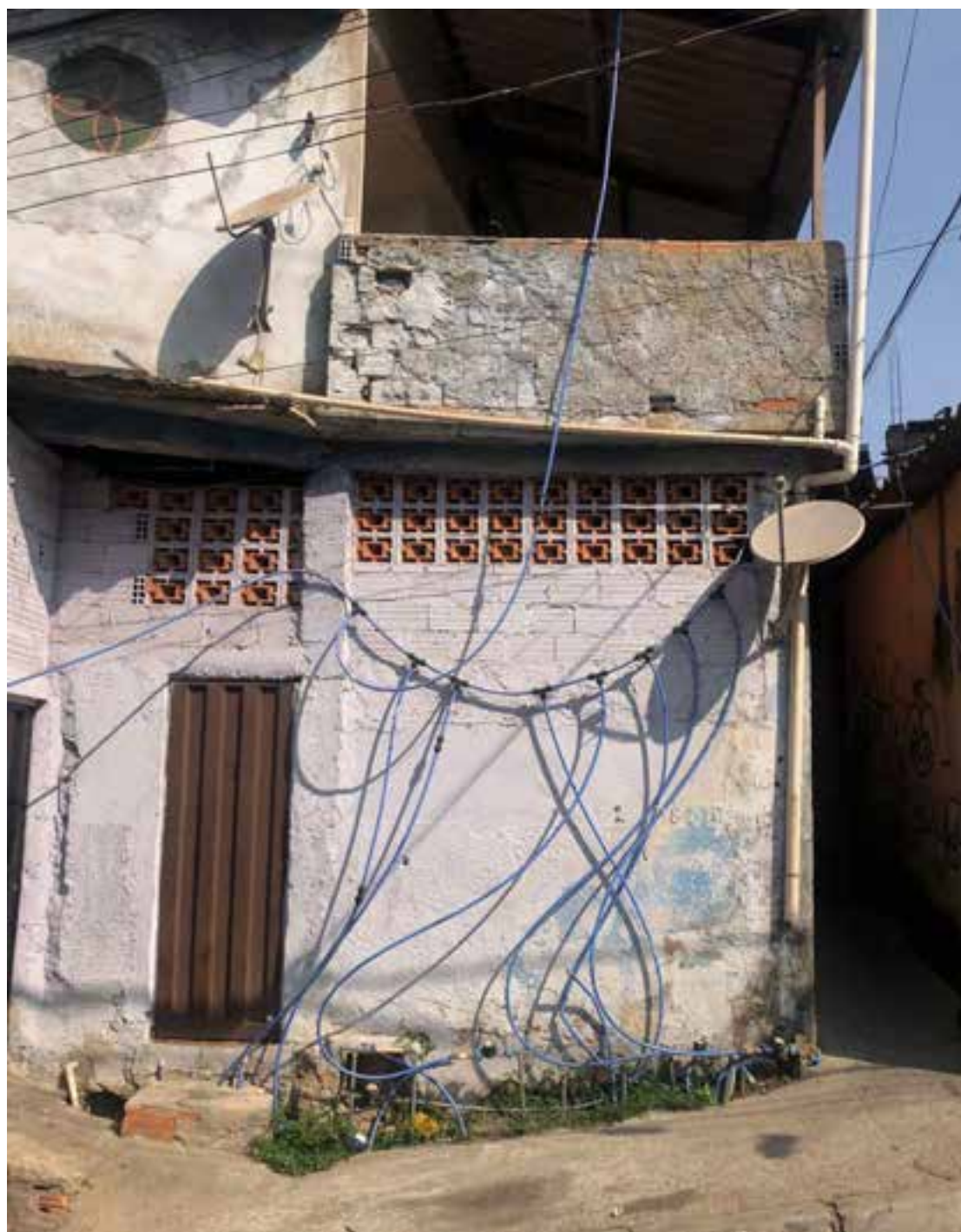
Fig. 3: Water connections exposed on a house facade at Pedreira Prado Lopes, in Belo Horizonte, a city located in the southeast of Brazil. Source: Author, 2022.
